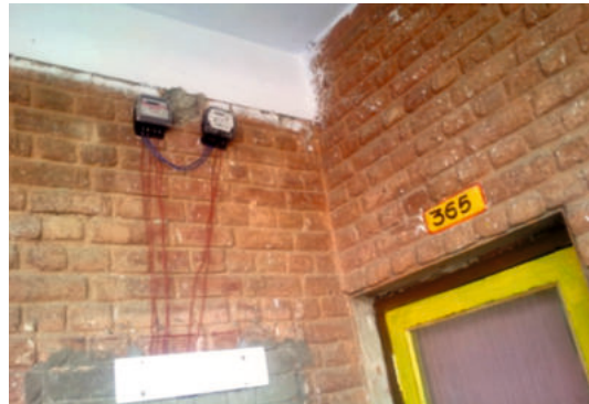
Figure 10: Electric metering to determine end use and total energy consumption at room level
