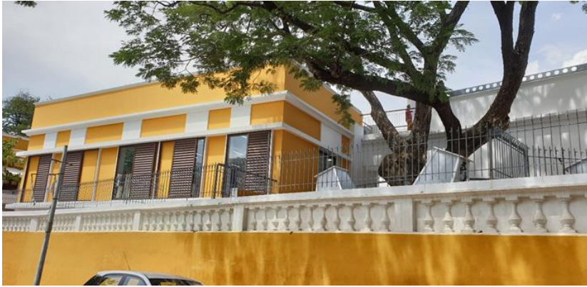
Figure 2: External facade as per heritage conservation guidelines -- with castellated beams and polycarbonate cones peeping out
