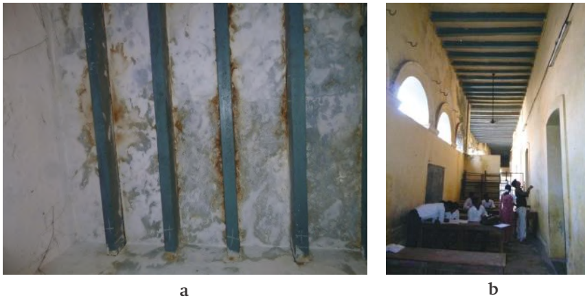
Figure 11:(a) Deterioration due to water seepage; (b) Verandah with later addition of Calve College (Image Credits – NCSHS, IIT Madras)
