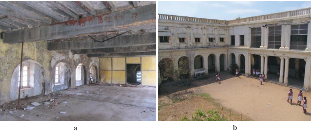
Figure 7: (a) Distressed beam in upper floor of Pensionnat de Jeunes Filles; (b) View of Courtyard of Pensionnat de Jeunes Filles (Image Credits – NCSHS, IIT Madras)
