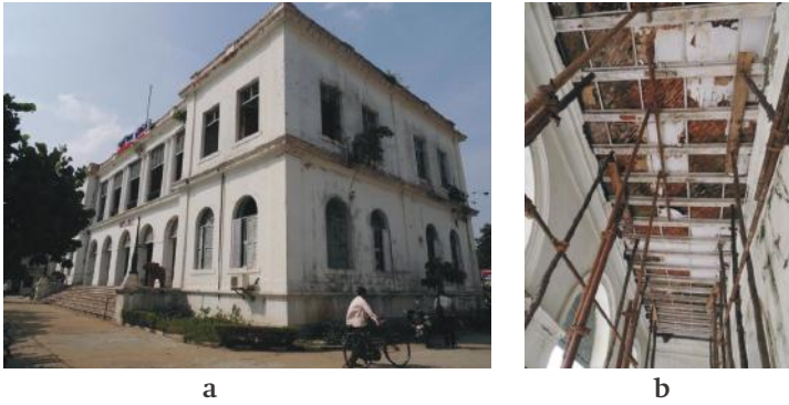
Figure 2: (a) La Mairie de Pondicherry before collapse; (b) Condition of verandah before collapse (Image Credits – NCSHS, IIT Madras)
