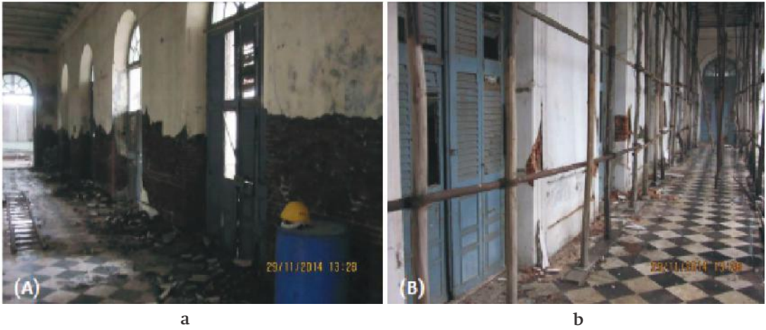
Figure 6: (a) Load bearing walls with partially removed plaster; (b) Delamination and bulging of plaster due to crushing failure. (Image Credits – INTACH Pondicherry)
