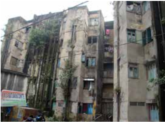
Figure 6: Dilapidated condition of a slum rehabilitation building at Chetla
